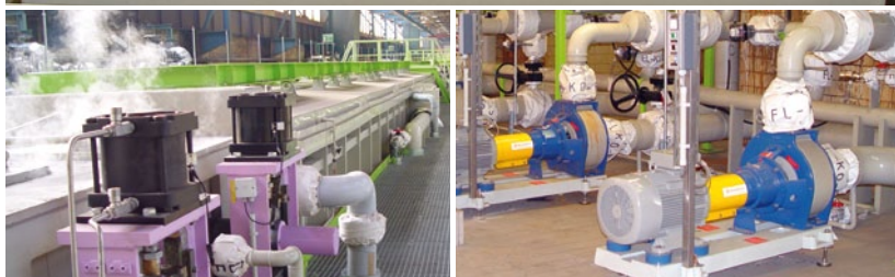
General view of the pickling line and the various tanks
