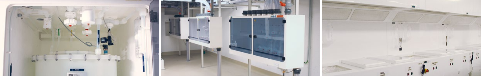
From left to right: interior view of the chemical supply system; distribution systems for equipment ports; manual wet bench
