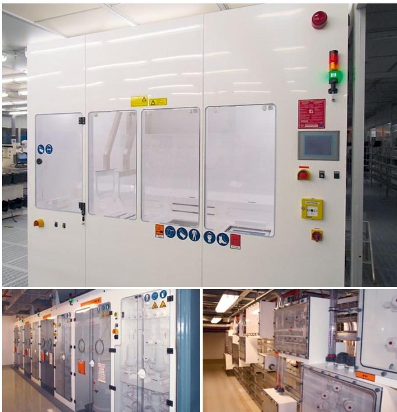
Top: automated wet-processing unit for the machining of silicon wafers; bottom left: fully automated supply systems for high-purity chemicals; bottom right: distribution systems for equipment ports
