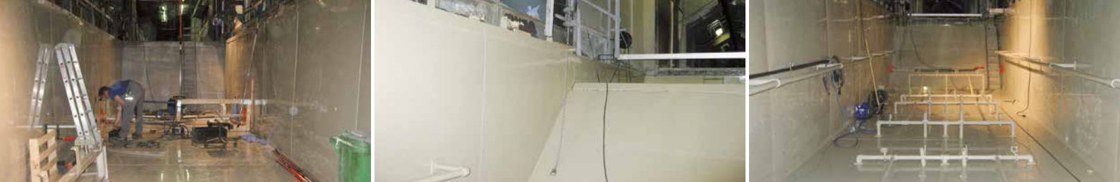
From left to right: applying the SIMONA® PP AlphaPlus® lining to the cathodic electrocoating bath; bath overflow; installing the nozzle pipes
